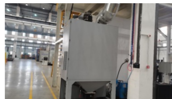
▶ Laser-cut waste gas treatment equipment
