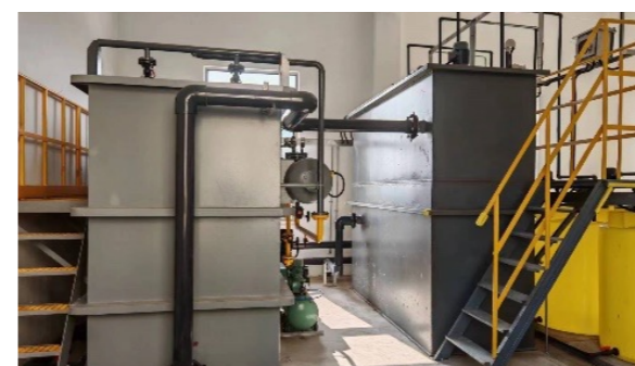
▶ New waste water treatment station
