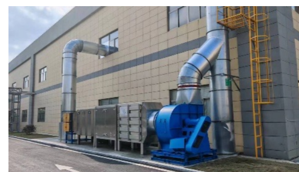
▶ New waste gas treatment equipment
